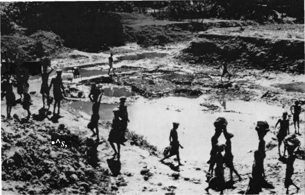
FIGURE 16.2. Workers Under the Test Relief Program Moving Earth to Reconstruct a Road (courtesy of Dr. R. A. Cash)
