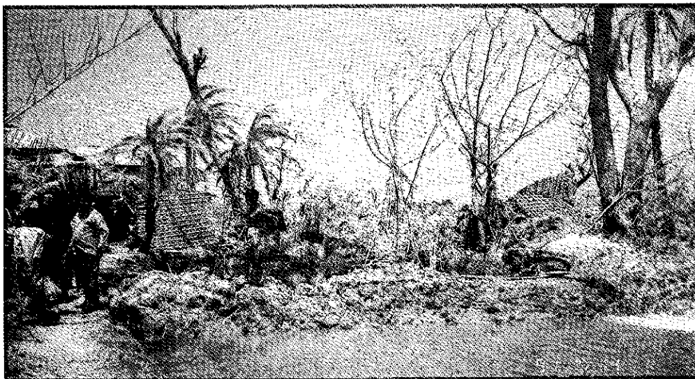
Rehabilitation of a pond in disaster-affected area. Restoration of the normal water supply situation.
