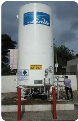
Existing Oxygen Liquid tank Secondary Source
